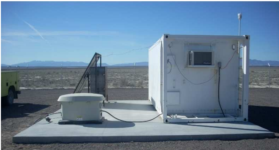
Figure 23: CLF (right). Solar-battery system (left back) is used to control and monitor. Liquefied petroleum gas generator (left front) whose controller is powered by solar-battery and switched remotely, is used to laser module and air conditioning.
