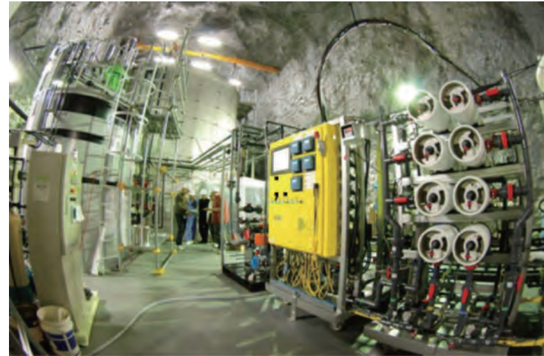
Figure 1: The EGADS facility. The 200-ton scale model of SK is in the back of the image, with the water filtration system in the foreground.
