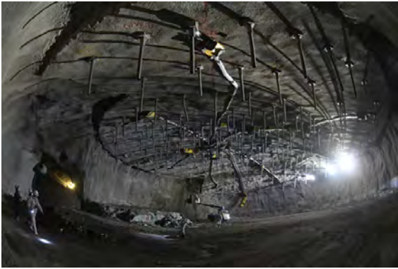
Fig. 38. The ceiling part of HK main cavern. The diameter in the picture is 40m, that will be extended to 69 m design diameter. Then the excavation will continue to go down to 70 m depth.
