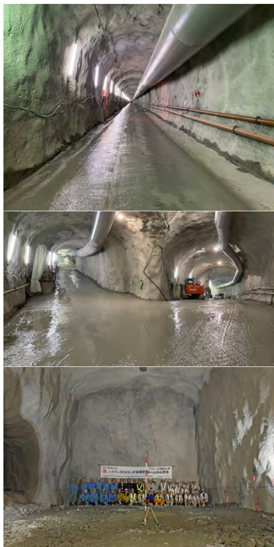
Fig. 37. The excavated access tunnel (top). The branch of approach tunnel toward top and bottom part of main cavern (middle). The center of HK dome reached on 23th, June 2022 (bottom).
