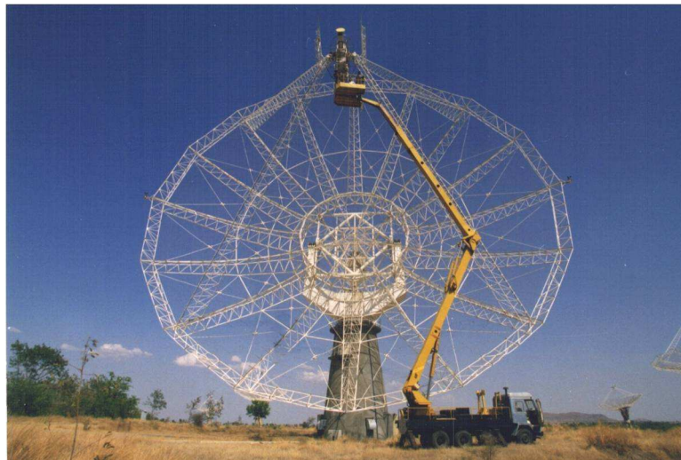
Figure 2. One of the 30 GMRT Antennas
