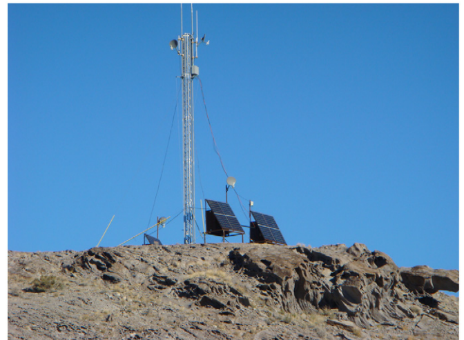
Fig. 5. The Smelter Knolls communication tower, one of three in the array. There are three stands each with four solar panels. Those stands contain batteries, data acquisition PC and network instruments for long distance link.
