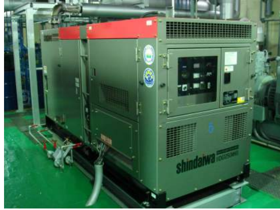
Fig. 2. A dynamo of 115KV.
