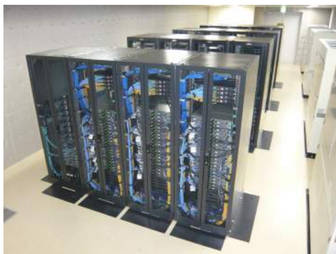
Fig. 1. Photo of the central computer facility in ICRR upgraded in 2014.
